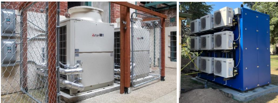
Figure 5. Two Heat2O units at Lassen Apartments, (left), and Waterdrop skid at Kings View Manor (right). Source: Association for Energy Affordability
